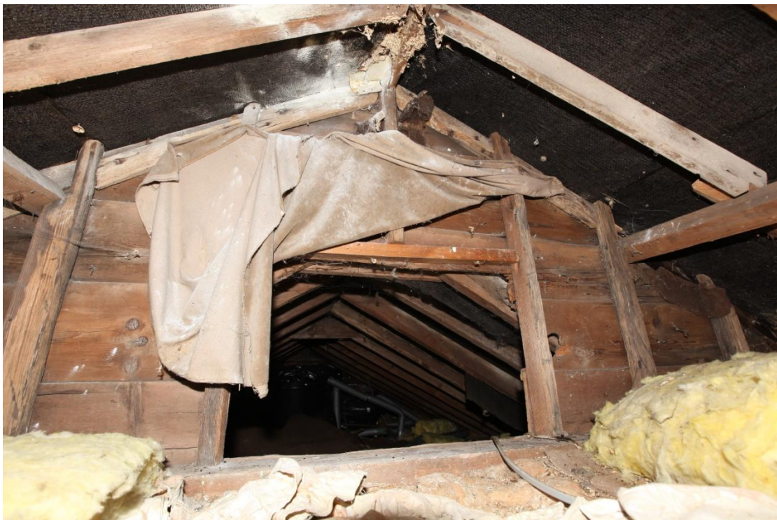
Illus. 16. The roof structure of the taller western section (2) showing the boarded studwork partition adjoining the lower section (1) to the east. The connecting aperture has been inserted by cutting the boarding. The softwood rafters of the eastern section are much the same but appear to lack purlins.
