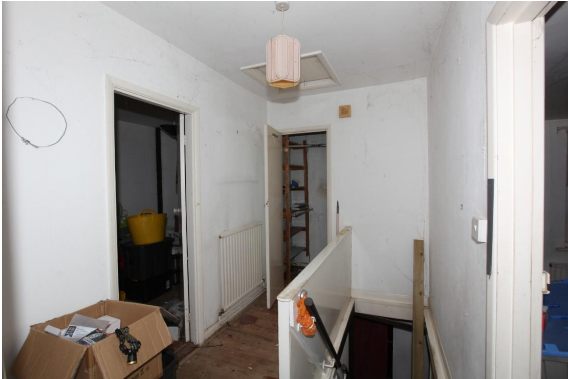
Illus. 13. The first-floor stair landing from the rear (south) showing its late-20th century plasterboard walls and architraves with the entrance to the western bedroom (2f) on the left.
