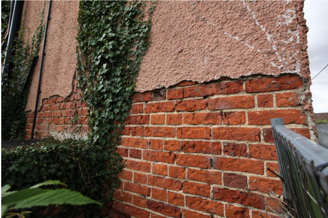
Illus. 4. A detail of the eastern external gable showing its high-quality red brickwork laid in what appears to be a form of Monk Bond beneath the modern cement render. The brickwork of the western gable exposed in the roof appears to consist of contrasting gault (white) brick (illus. A2. 15).
