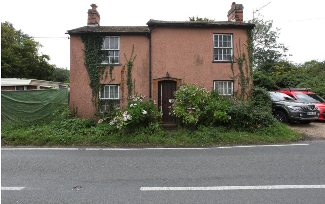
Illus. 2. The unusually asymmetrical northern facade with uniform mid-19th century sash windows without horns to their corners (as would be expected in the late-19 th century). The brickwork is entirely concealed by 20 th century cement render and it is unclear whether the lower section of the building on the left (1) represents a slightly later addition to the taller section on the right (2).
