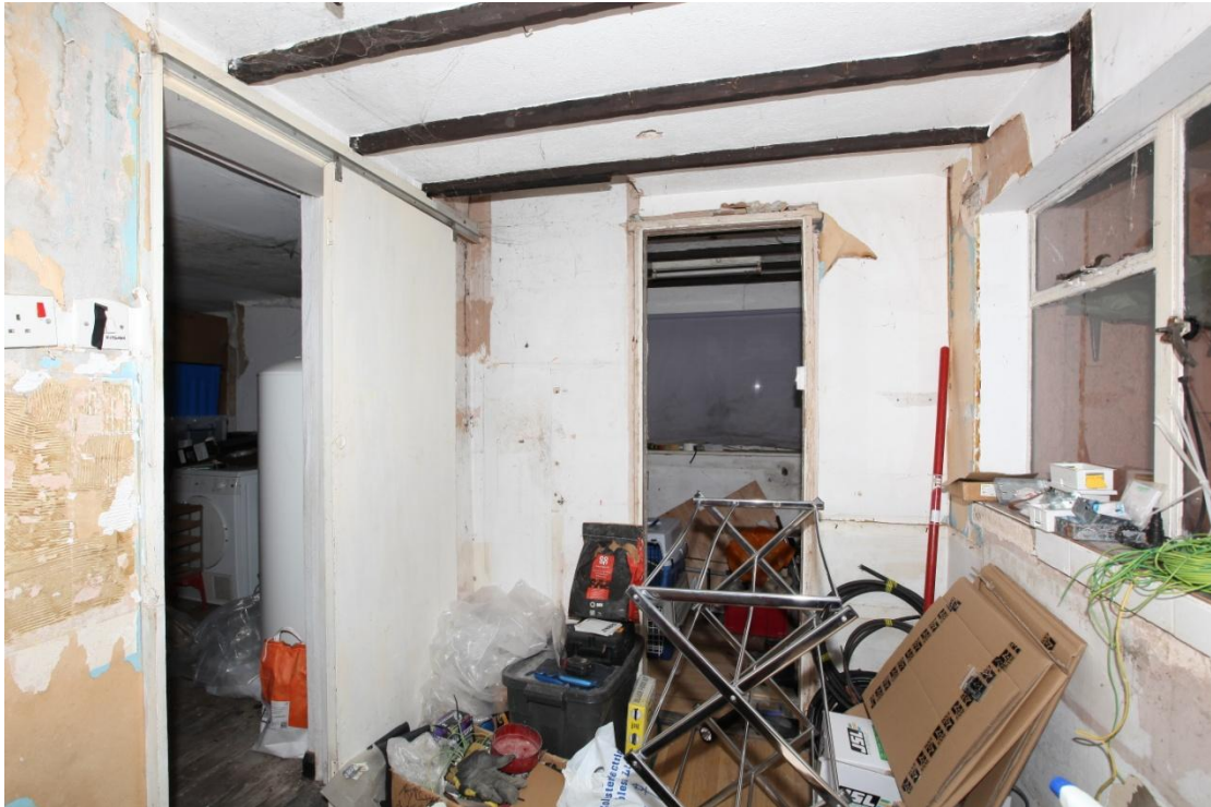
Illus. 9. The interior of the mid-20th century kitchen extension (3) from the east showing its southern Crittall window on the right with the door to the dining room (1) on the left. The ceiling joists appears to have been exposed from the outset to create a Mock Gothic appearance.
