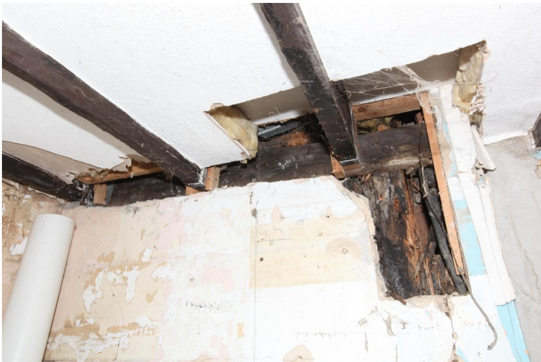
Illus. 10. A detail of the exposed softwood studwork of the original rear wall in the northern interior of the kitchen extension (1). It appears that the entire back wall consisted of rendered studwork in contrast to the more expensive brick of the northern facade and gables.
