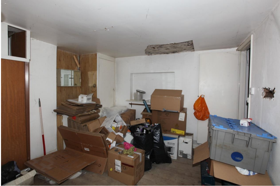
Illus. 11. The southern interior of the eastern bedroom (1) showing the recess of the original rear window blocked by the 20 th century extension (3) with the door to the stair landing on the right. There is no evidence of a fireplace in the eastern gable to the left and the narrow chimney served only the ground floor.
