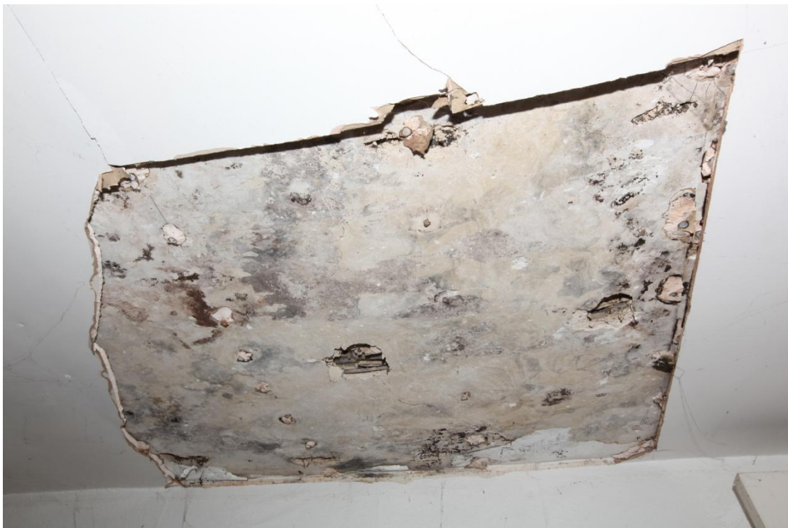
Illus. 12. A detail from the north of the original lath-and-plaster ceiling of the western bedroom (1f). The coarse lime plaster is typical of the 19 th century, but was hidden by plasterboard during the late-20 th century refurbishment.
