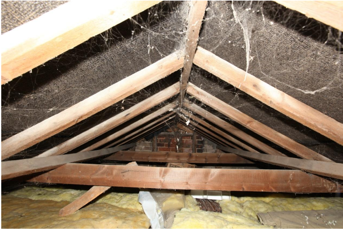
Illus. 15. The original softwood roof structure of the taller western section (2) looking towards the apparent gault-brick fabric of the western gable with the red-brick chimney in the centre. The edges of the gault brickwork appear to be broken suggesting the present chimney may be represent an alteration.
