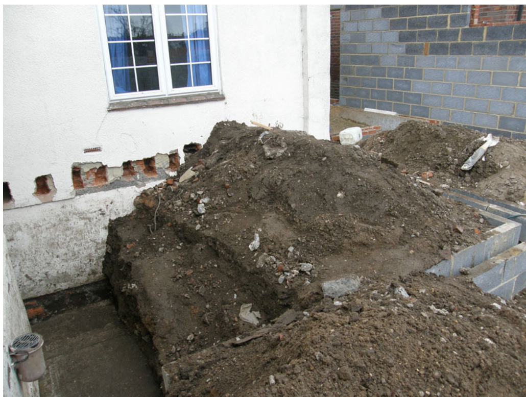
Photograph 1 Photograph showing depth of soil to be moved and sifted for bone. The breeze-blocks in this photograph show where the foundation trenches had been dug.
