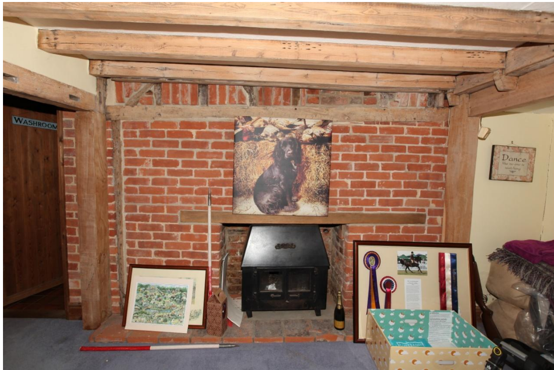
Illus. 7. The modern brick fireplace in the western gable of phase 1 showing the original mid-rail with a diagonal primary brace to the left. Some studs appear to be pegged to the rail, although the timber may have been re-used, but most are not. The posts to left and right relate to the mid-20 th century restoration (phase 2), as does the re-used southern mid-rail on the left.
