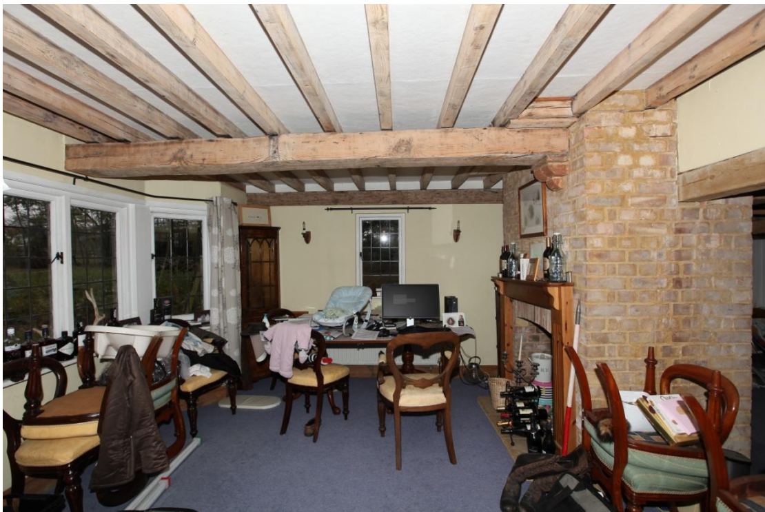
Illus. 10. The interior of the north-eastern extension (2) as seen from the west, with its original chimney containing identical back-to-back fireplaces adjoining bay 1b on the right. The tall-sectioned pine ceiling joists have been cleaned of their original Mock Tudor stain, and are lodged on an axial joist in the same crude manner as those of the contemporary ceiling in phase 1.
