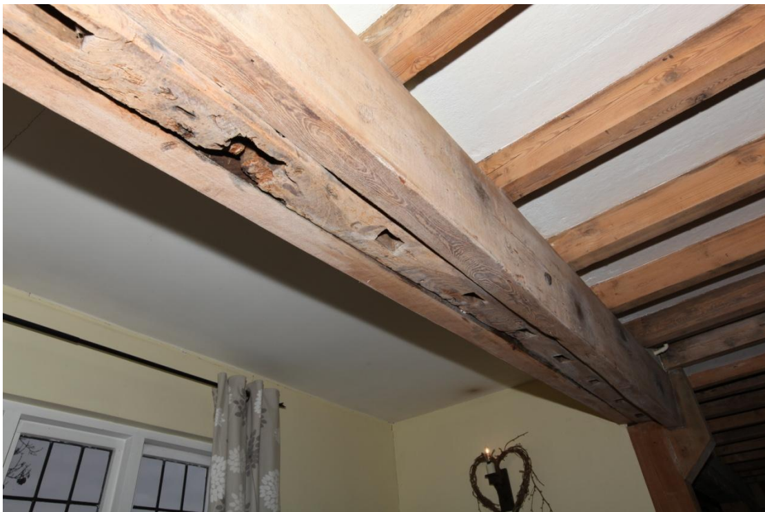
Illus. 6. A detail of the front wall of the eastern bay (1b) showing the empty, unpegged mortises of its original mid-rail from which the ground-floor studs have been removed. The timber is now supported by a pair of bolted clamps where it adjoins the lean-to extension (4c).
