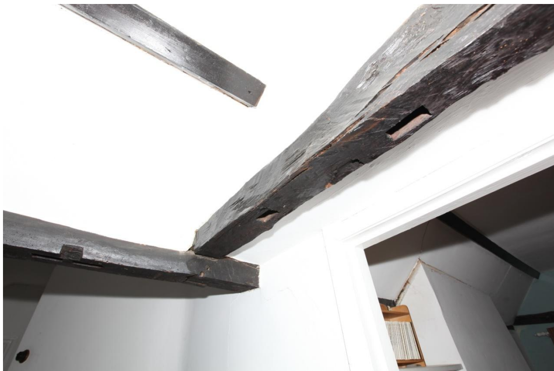
Illus. 12. A detail of the central tie-beam in illus. 11 showing the empty, unpegged stud mortises of the first-floor partition which divided the building's two original bays. Identical empty mortises are visible in the roof-plate (left) along with empty stud notches, indicating more than one significant phase of rebuilding.
