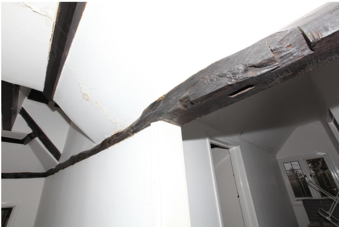
Illus. 14. The northern roof-plate of the original western bay (1afl) showing its combination of empty notches and unpegged mortises. The mortises are likely to relate to the original wall studs which were later replaced by a series of notched and nailed studs – most of which were renewed in turn during the 20 th century restoration. Note that the western gable tie-beam in the rear to the left is at the same level as the roof plate, with an iron strap securing the two in a manner rarely found before the 1830s.
