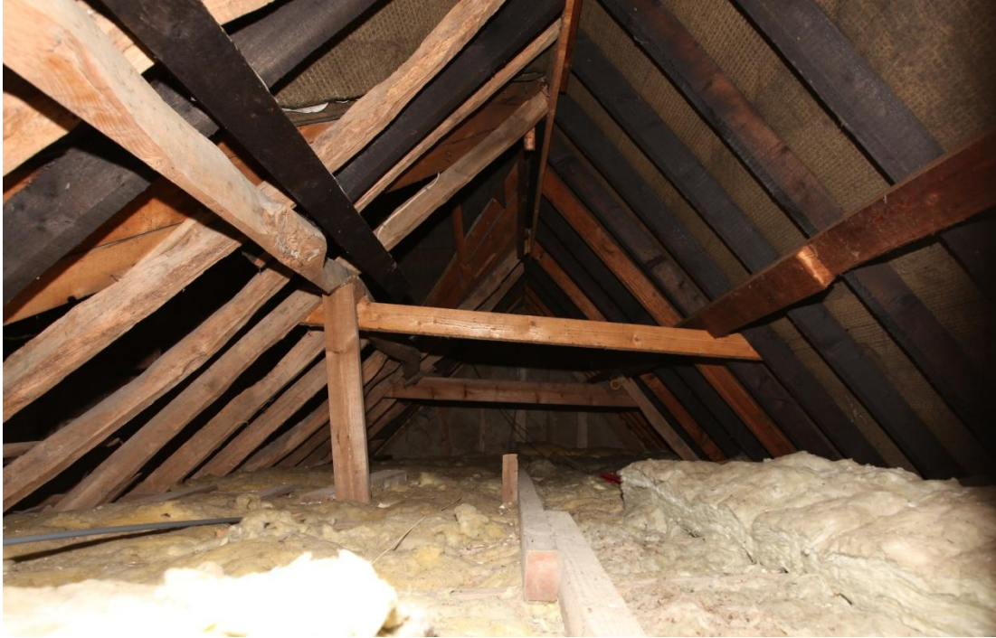
Illus. 15. The original roof structure of phase 1 seen from its western gable. The waney, unpainted rafters on the left (north) are original but the collars and the southern rafters are 20 th century replacements in two phases – one set of new softwood timber has been stained black, presumably with preservative. The studs of the eastern gable appear to be original indicating the building was initially hipped at only one end.
