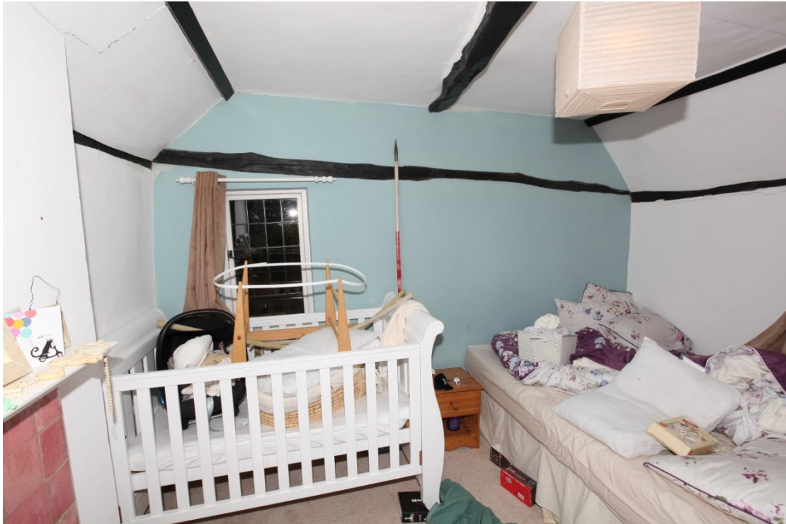
Illus. 13. The eastern internal first-floor gable of phase 1 (1bf) showing the original tie-beam with a central mortise for the axial joist of a missing original ceiling at eaves level. Identical mortises are visible in the centres of all the exposed tie-beams.
