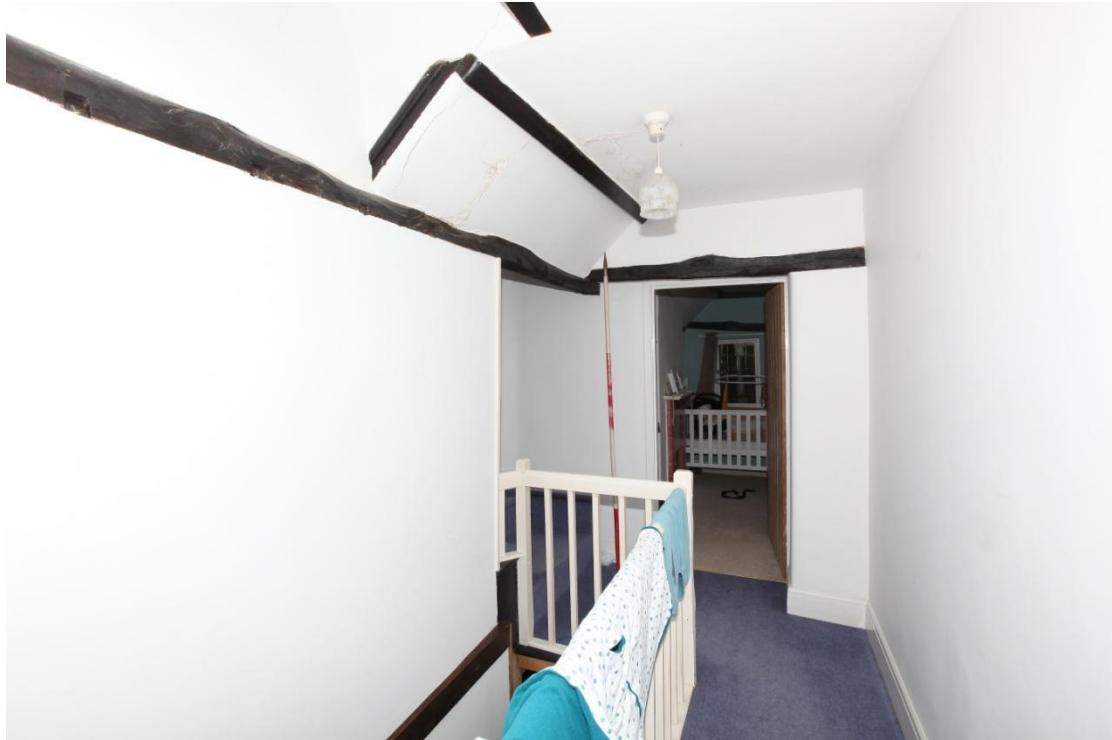
Illus. 11. The first-floor stair landing (1afl) from the west showing the black-painted original northern roof-plate and central tie-beam of phase 1, with the bedroom above its eastern bay (1bf) in the rear. Note the empty notches for studs in the roof-plate (top left), which suggest the wall fabric has been renewed twice.
