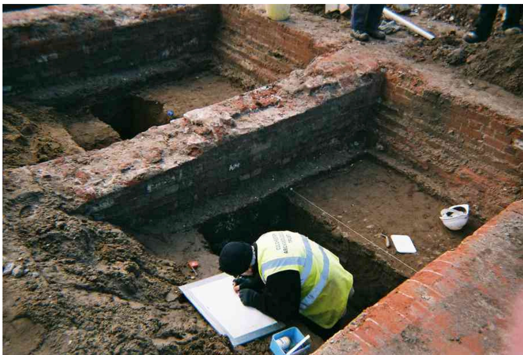
Plate 15.1 Brick foundations of the military prison foundations over the Iron Age dyke (R Masefield).
